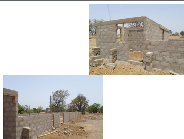
Construction of the animal pen, storage building and office at the Trax-Kavli Scholarship Farm
